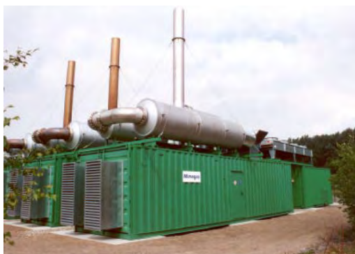
Plant "Kurl Shaft III"
